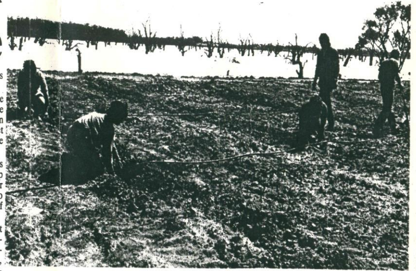
MANY HANDS MAKE LIGHT WORK: With help from two volunteer groups, local community members and the Barmera-Moorook Field and Game Reserve, work on the Loveday Evaporation Basin is nearly completed. The second group of the Australian Trust for Conservation volunteers planted more than 1300 native trees and add the finishing touches to one of the sections. The group is also partly responsible for the erection of a rabbit-proof fence and the installation of a drip irrigation system.
